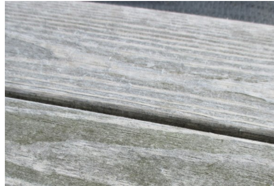
Natural occurring surface fibres on decking.
